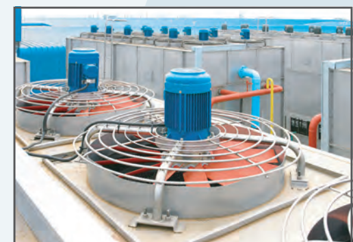
Fan and water pump
