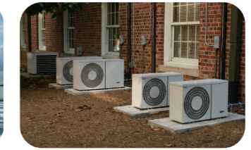
Air Conditioning System
