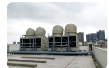
Circulating water in HVAC
