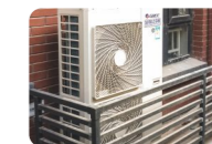
Air conditioning system
