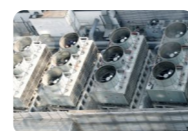
Air conditioning system
