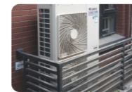
Air conditioning systems
