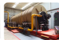
Gas boiler hot water Circulation
