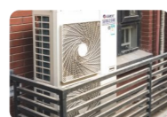
Air conditioning Secondary systems
