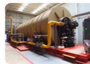
Gas boiler hot water circulation
