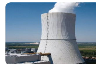
Circulating water in cooling tower
