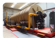
Gas boiler hot water circulation
