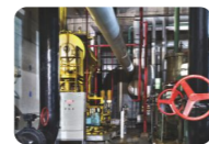
Indoor pipeline circulation
