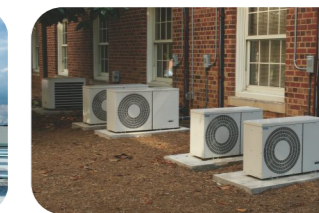
Air Conditioning System
