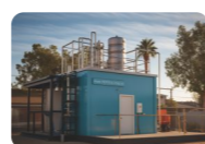
Hot water boilers
